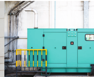
POWER BACKUP (DG)
